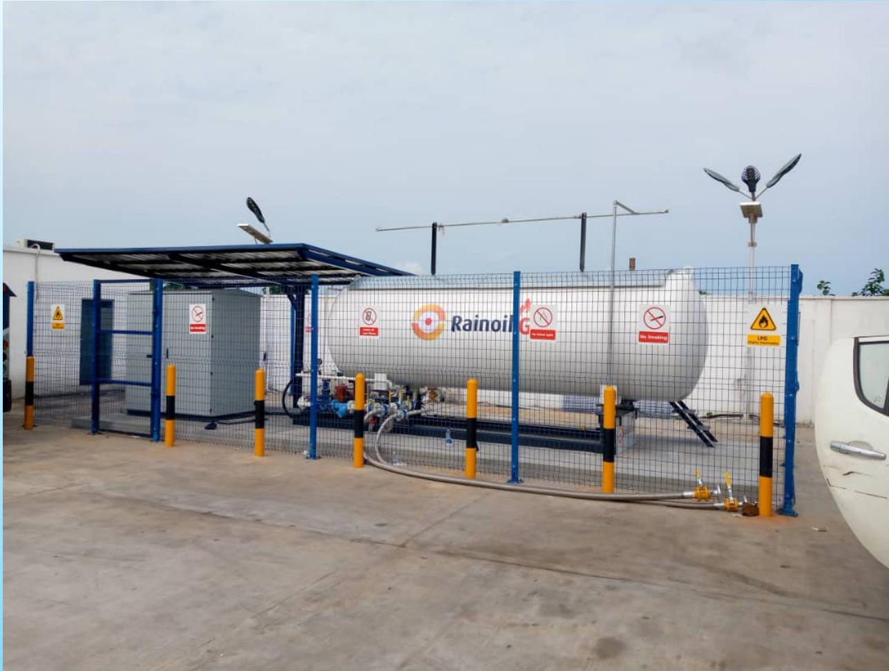
LPG SKID BRANDING
